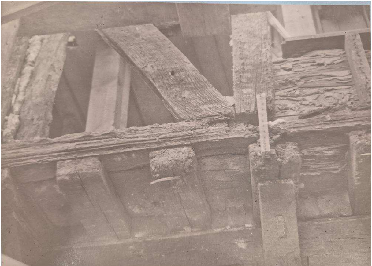
Figure 22 Photo taken in 1937 during removal of render exposing timber framework and jettied section. 52
