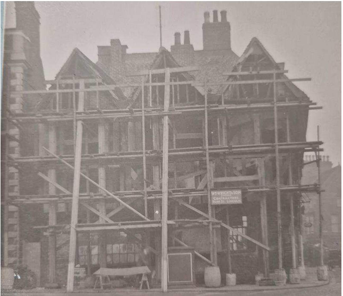
Figure 19 Photo taken in 1937 during works with scaffolding up and render stripped to reveal the timber framework. 49
