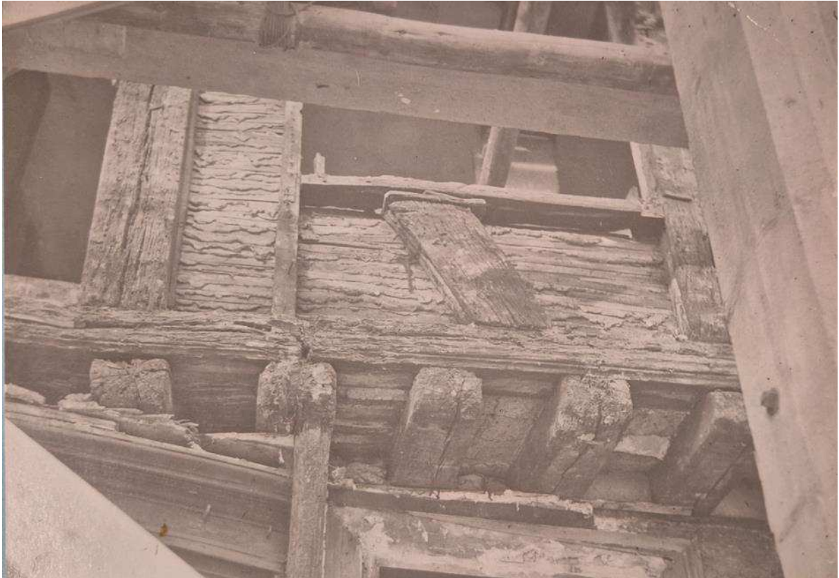
Figure 21 Photo taken in 1937 during removal of the south elevation render exposing some of the timber framework and the back of surviving internal plasterwork above jettied section and window opening. 51
